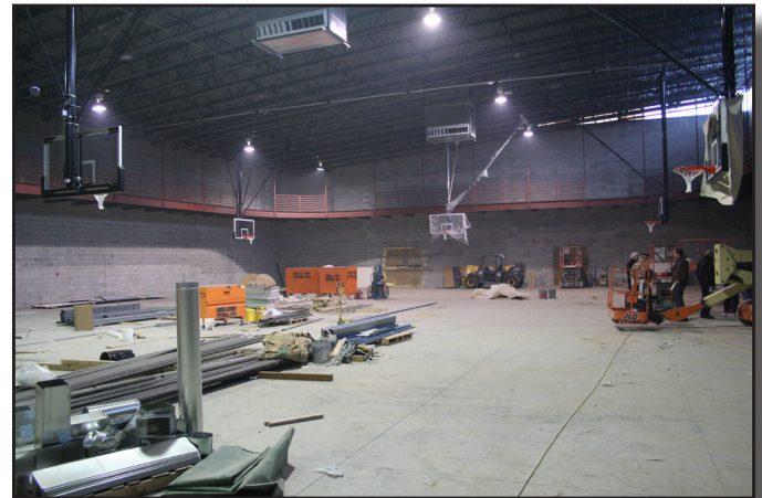
The main gymnasium of the facility will feature two basketball courts and a walking track.
